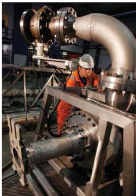
Riserless mud recovery (RMR) technology reduces pollution and environmental impact by controlling handling and disposal of drill cuttings (Fig. 1; photo provided by Ability Subsea AS).
